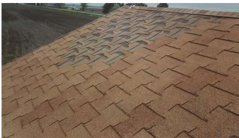
Example of Wind Damage
