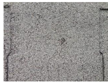
Hail damage close May 26th
